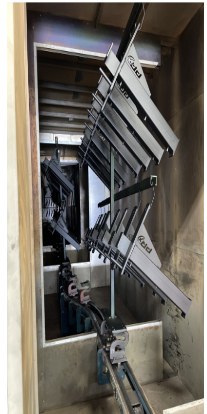
Photo: Powder Coating Oven
